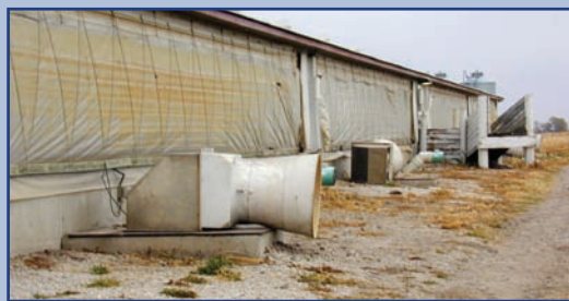
Manure Pit Fans and Side Curtains
